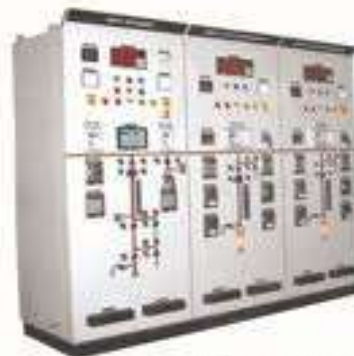
Figure 7 RELAY & CONTROL PANEL
